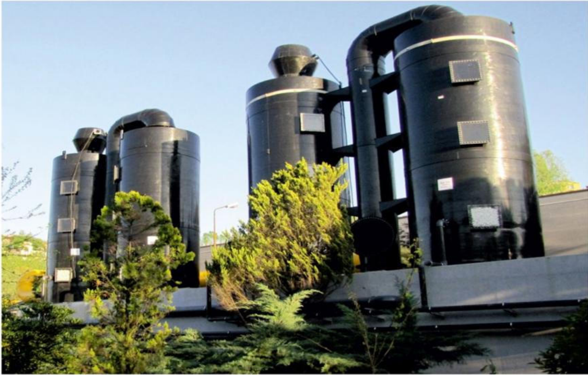
WET SCRUBBER SYSTEM - HDPE BODY BALTIMANI İSKİ - İSTANBUL / TURKEY
