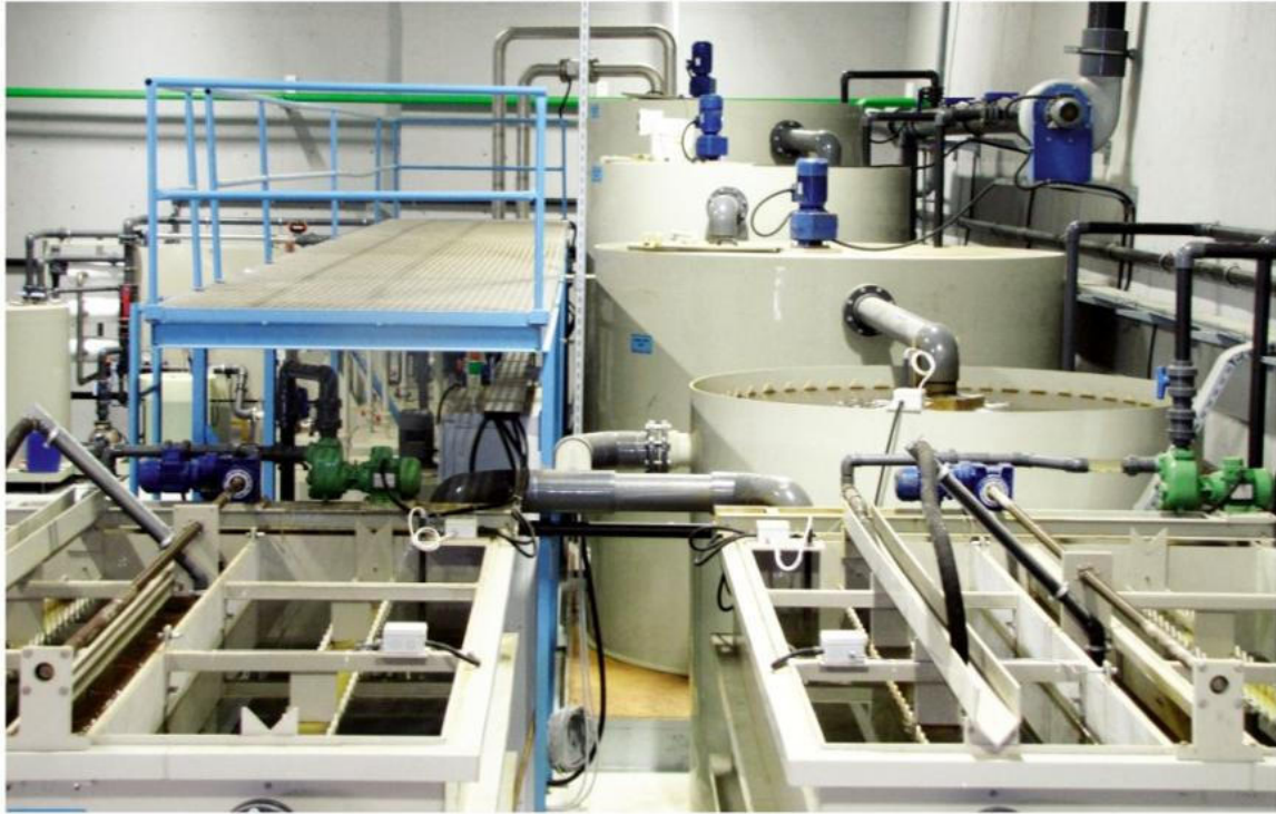
TEXTILE WASTEWATER TREATMENT MARTUR - KÜTAHYA / TURKEY
